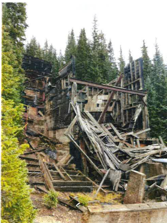
Figure 2. Dilapidated hazardous middle portion of the mill building, probably not worth saving except for concrete foundation.
