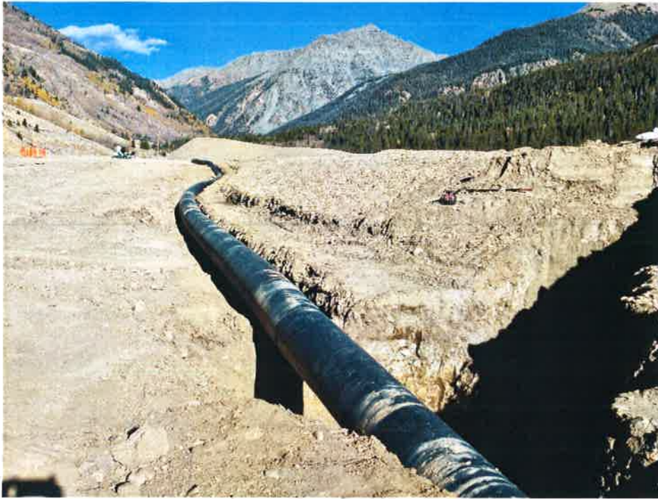
View looking northeast of leachate drainage system, 24" HDPE pipe, in trench prior to burial
