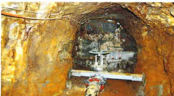
Red and Bonita Bulkhead with flow-through pipe and valve
