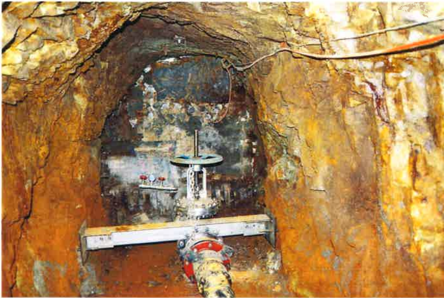
A bulkhead was installed at the Red & Bonita Mine in 2015. The EPA next week will temporarily close the valve for a short-term monitoring project.
