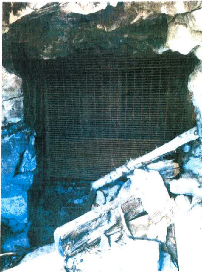
Photo #2. Gary Owen Tunnel Portal 2021 – Note lower left side under gate where trespassers have dug under gate to gain access. Gate installed by Colorado DMG in 2008.
