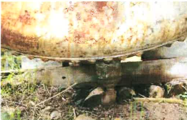
Bottom end drain (original or added?)
