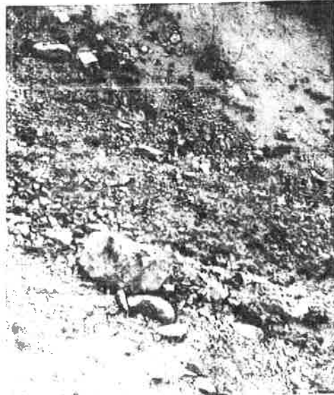
Collapsed mine portal (circle 1)
