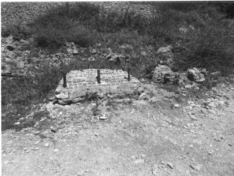
5SA407. Compressor mount to the left with the probable electric motor mount to the right, looking north-northwest. Photo by Jon Horn, 6/20/2023.
