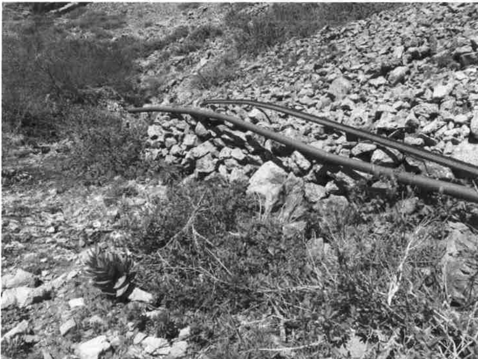
5SA407. Looking west at the central retaining wall remnant with ore car rail and compressed air pipe disposed on it. Photo by Jon Horn, 6/20/2023.
