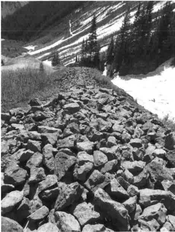
5SA407. Downslope view of the southern avalanche deflector wall, looking east-southeast. Photo by Jon Horn, 6/20/2023.
