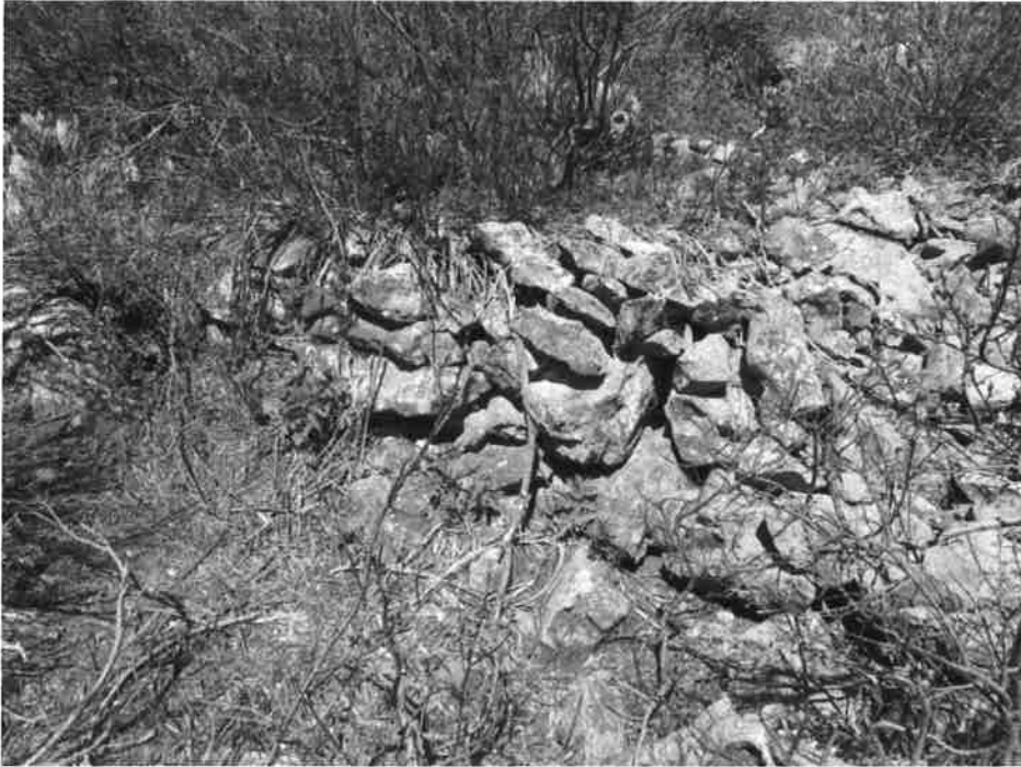
5SA407. Looking west at the southernmost retaining wall. Photo by Jon Horn, 6/20/2023.
