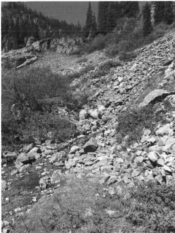
5SA407. Collapsed adit with exclusion gate and post and plank framing debris, looking west. Photo by Jon Horn, 6/20/2023.
