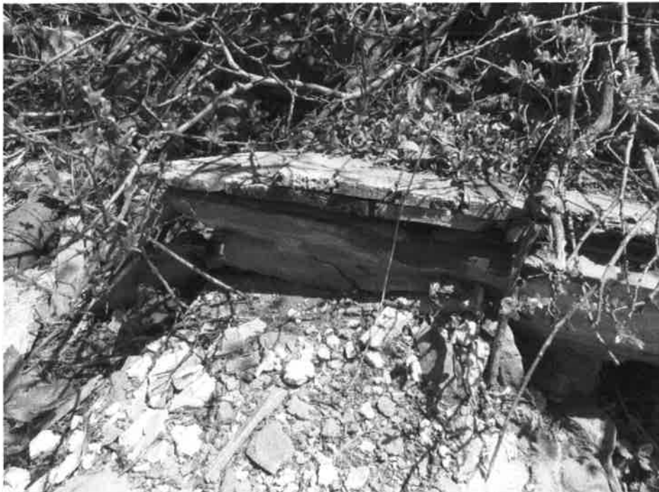
5SA407. Building floor remnant showing diagonal 1-x-6-in. subfloor topped by 1-x-4-in. tongue and groove flooring set on 3 by 6-in. joist. View is to the north. Photo by Jon Horn, 6/20/2023.
